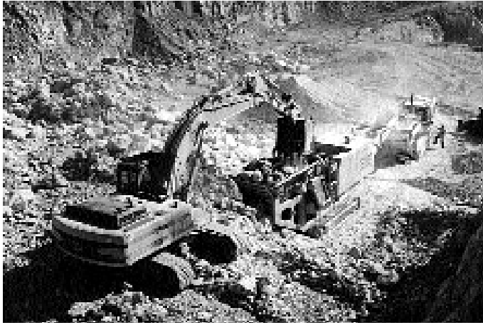
32 HQ Squadron work at Caravica Quarry – a heavy crawler excavator loads stone into a crusher.
